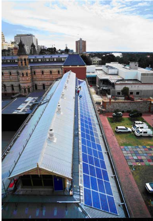
Photovoltaic installation on the South Australian museum
